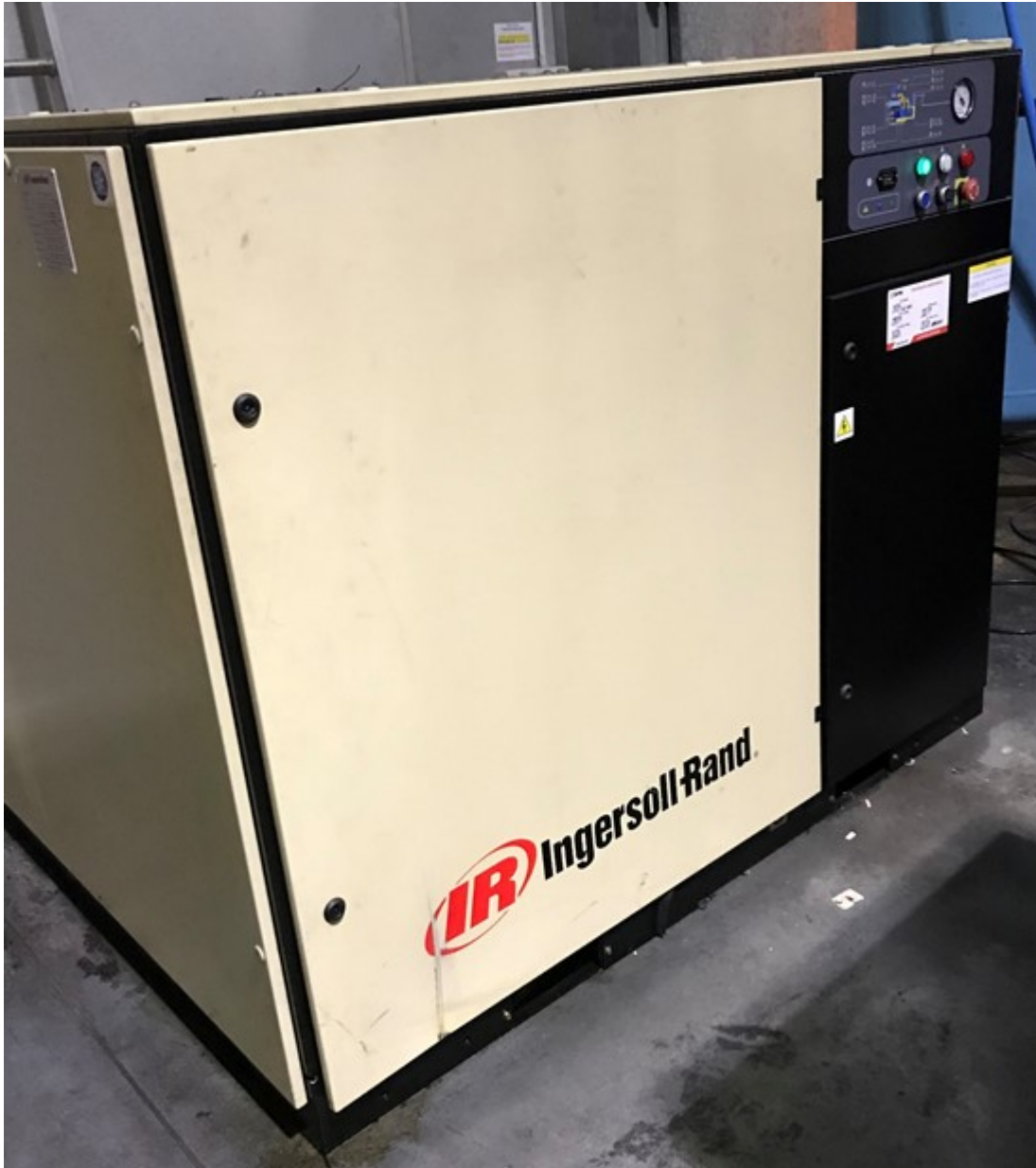
Figure 1 Tripping Ingersoll-Rand 70 kW Screw Compressor
