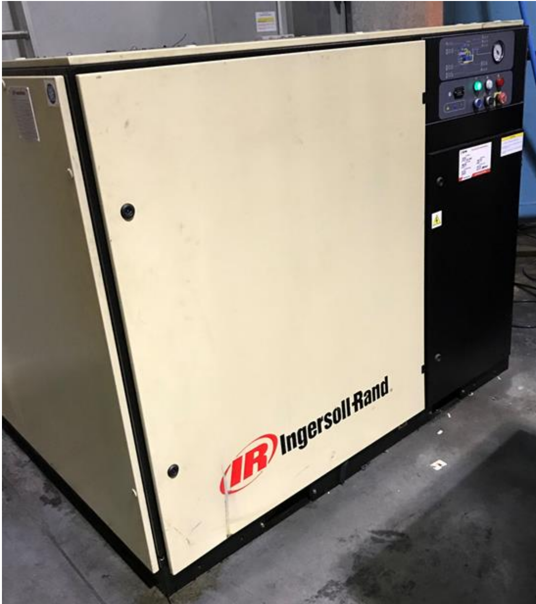
Figure 1 Ingersoll-Rand 70 kW Screw Compressor (the tripping one)
